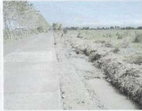
Pic 5.1 A scoured right shoulder of the San Leonardo - Jaen road which was 0.5 m underwater bet. Nov 30 to Dec 02, 2004.
