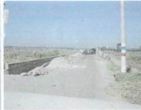
Pic 20.1 Eroded shoulder along the Baliuag - San Luis road that went underwater during Winnie & Yoyong.
