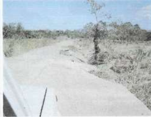
Pic 7.0 The Palayan - Natividad road in Bgy. Atate, Palayan went about 0.5 m. underwater at the height of T.D.Winnie.
