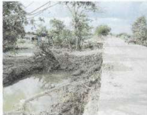
Pic 16.0 Floodwaters scoured the right shoulder of Zaragoza - San Antonio road at Bgy. San Francisco, San Antonio, N.E.
