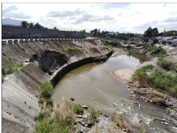
(Pic 66, above) A scoured slope dike protection along Lucung River in Concepcion, Tarlac which gave way at the height of Paeng’s generated river flow of the said river.
