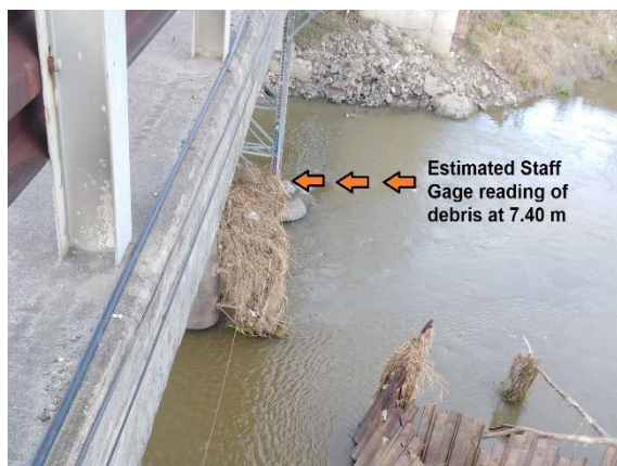
(Pic 67, above) Debris still clinging to the staff gage at Arayat station showing a reading at around 7.40m.
