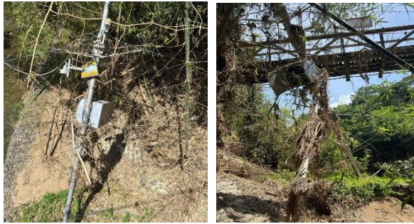
(Pic 42, L) The picture shows a destroyed monitoring system (CCTV and WLMS) of the Bulacan PDRRMO along Biak na Bato River in San Miguel that went underwater early morning of Sept 26. (Photos courtesy of Bulacan PDRRMO)
