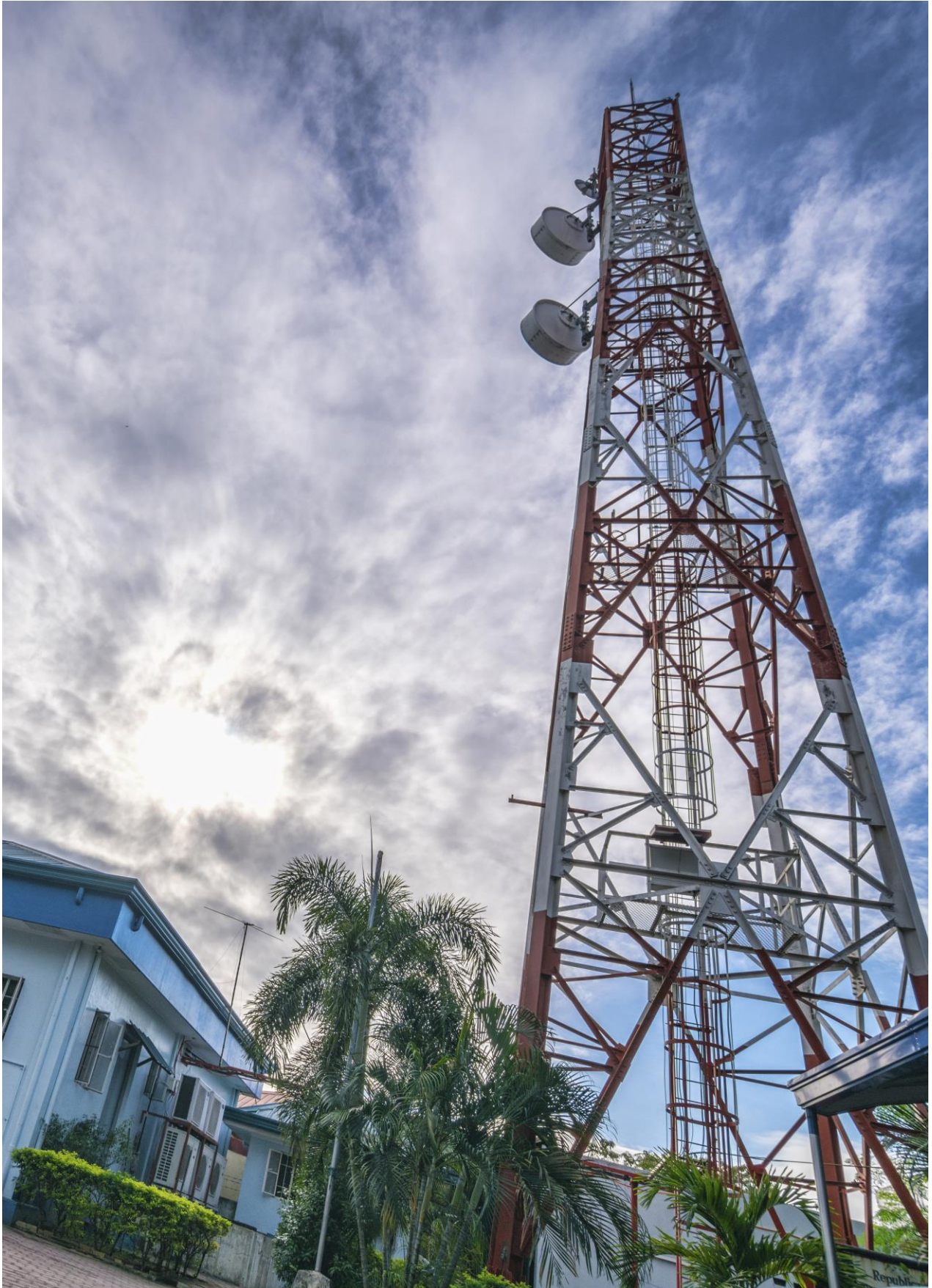
The PRFFWC Telemetry Tower within the PRFFWC compound located in DMGC, Bgy. Maimpis, CSFP
