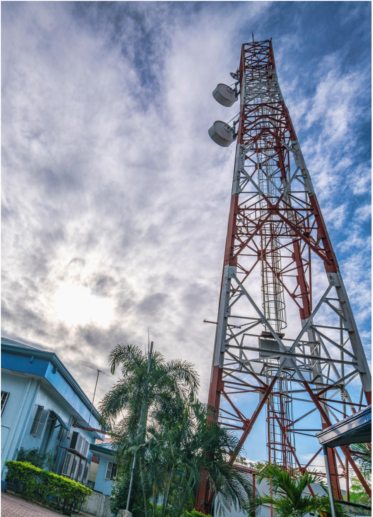
The PRFFWC Telemetry Tower located in the City of San Fernando, Province of Pampanga.
