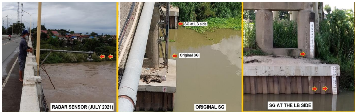
Pic 4 (below from L to R) the radar sensor installed March 2021 but operationally started July 2021; (below Middle) location of the original SG in the said stream gaging point; (below R) a SG placed on the bridge’s pier on the LB side of the river channel.
