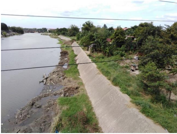
(Pic 16, left) A view of the concrete lined dike on the right bank (RB) of Angat River as seen downstream from the Plaridel-Pulilan Bridge.
